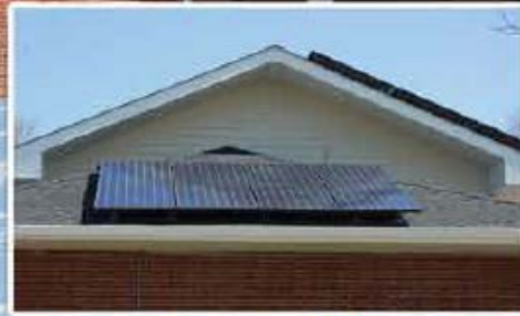
Solar panels installed on Garden City Park Water District administration building will help conserve energy and lower operating costs.
